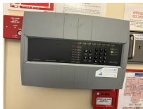
Fire Alarm panel no faults
