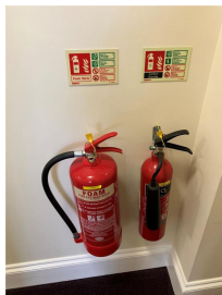
Fire extinguishers on hooks with clear signage
