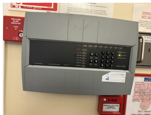
Fire Alarm panel no faults
