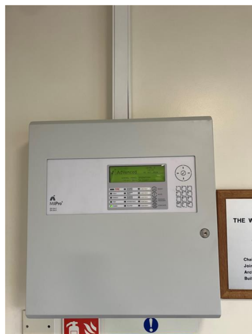
Fire alarm free from faults
