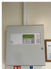
Fire alarm free from faults
