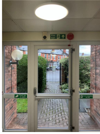
Fire exit push bar fully operational
