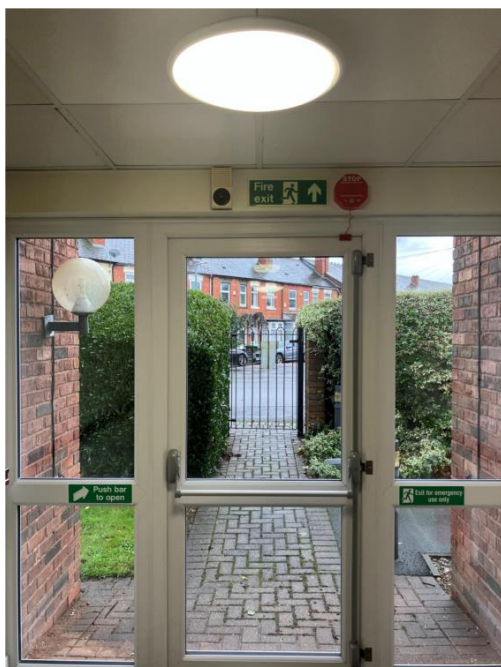
Fire exit push bar fully operational
