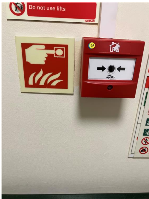
Fire alarm call point clear signage
