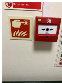
Fire alarm call point clear signage
