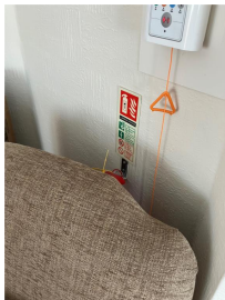
Fire extinguisher obstructed
