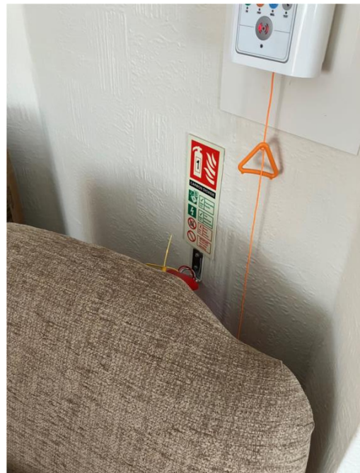
Fire extinguisher obstructed
