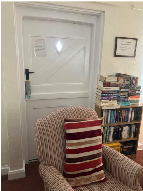
Fire Exit obstructed
