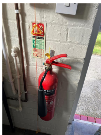
Fire extinguisher on hook
