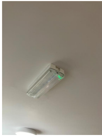
Emergency lighting installed
