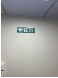
Fire escape route clearly indicated
