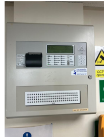
Fire Alarm panel no faults
