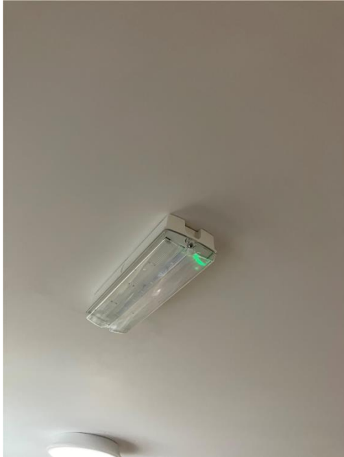
Emergency lighting installed
