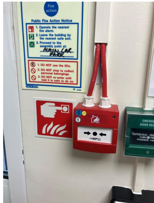
Fire Alarm call point clear signage
