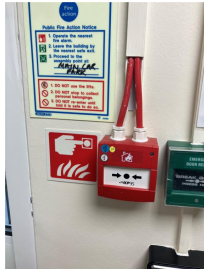
Fire Alarm call point clear signage
