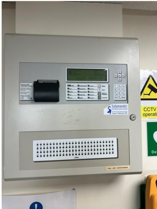
Fire Alarm panel no faults
