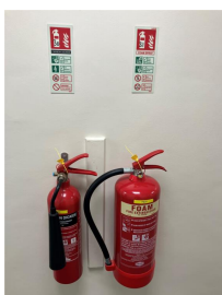
Fire Extinguishers on hooks with suitable
