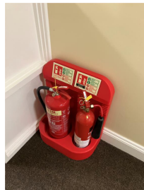
Fire Extinguishers on suitable stand
