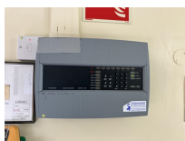
Fire Alarm panel no faults
