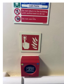
Fire Alarm call point clearly indicated
