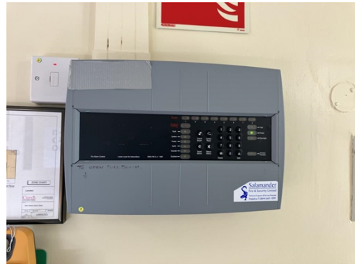
Fire Alarm panel no faults
