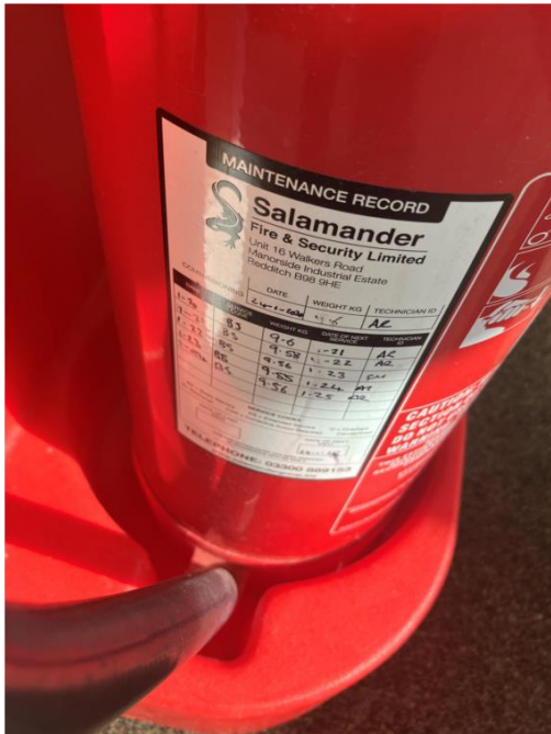
Fire extinguisher service 18-01-2024
