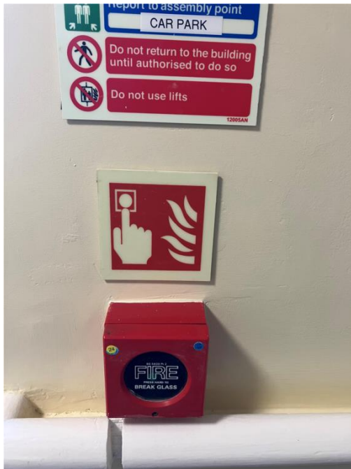
Fire Alarm call point clearly indicated
