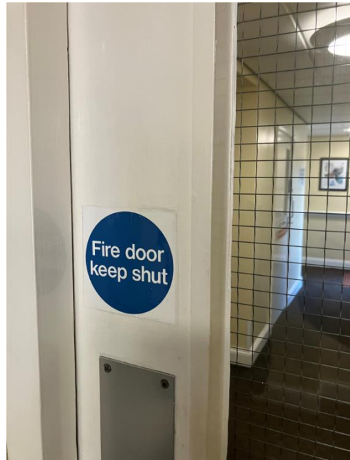
Fire door appropriate signage
