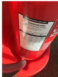
Fire extinguisher service 18-01-2024
