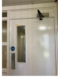
Fire Door self closers seen
