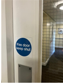
Fire door appropriate signage
