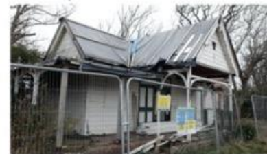
PAVILION WITH REPLACEMENT POSTS & CLOCK MISSING
