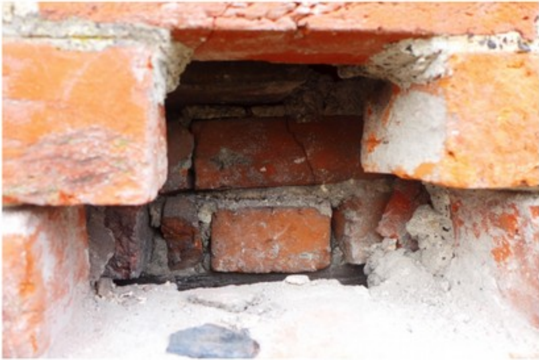
3. Sample opening up at front pier showing debonded outer leaf brickwork
