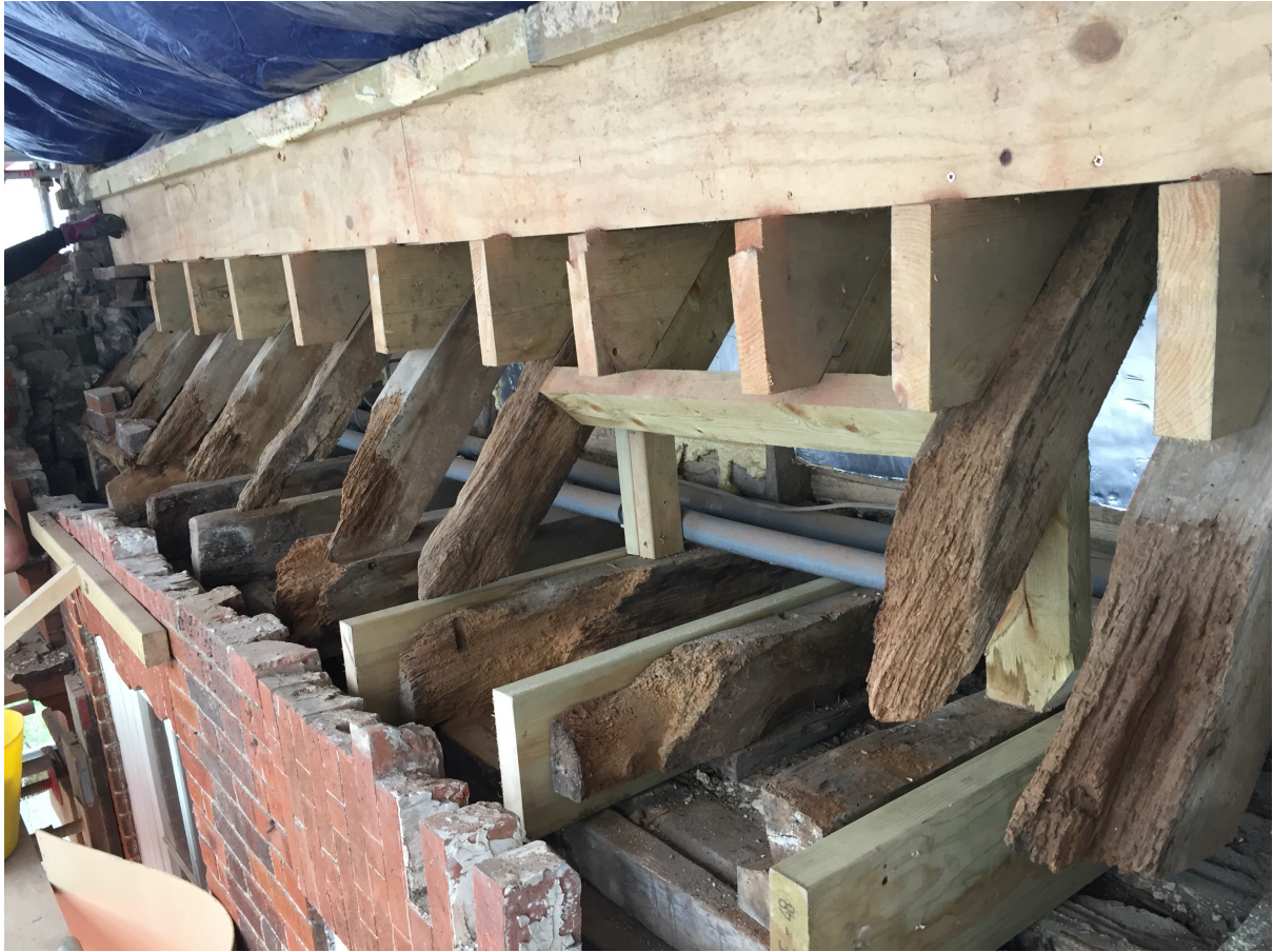
Timber decay within parapet structure
