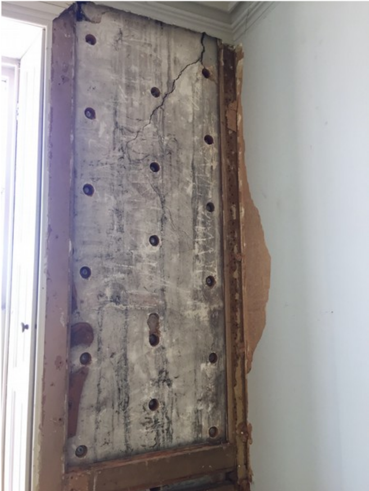
Following insertion of CINTEX anchors from internally note removal of linings to gain access to internal wall
