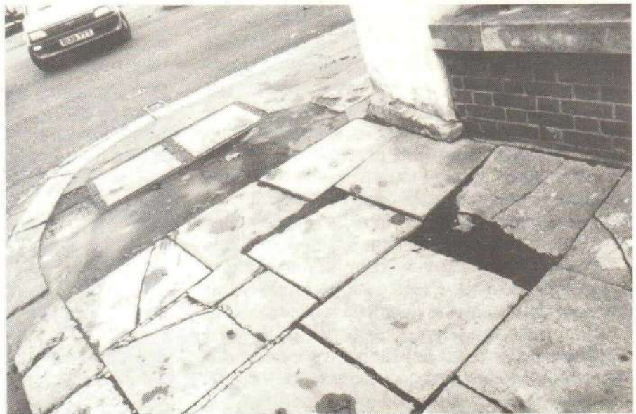
Damage to pavement at the corner of Ennismore Gardens and Kensington Road.
