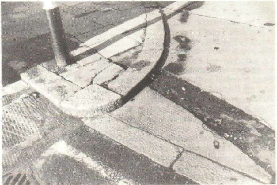
State of the pavement and highway between Trevor Square and Lancelot Place.
