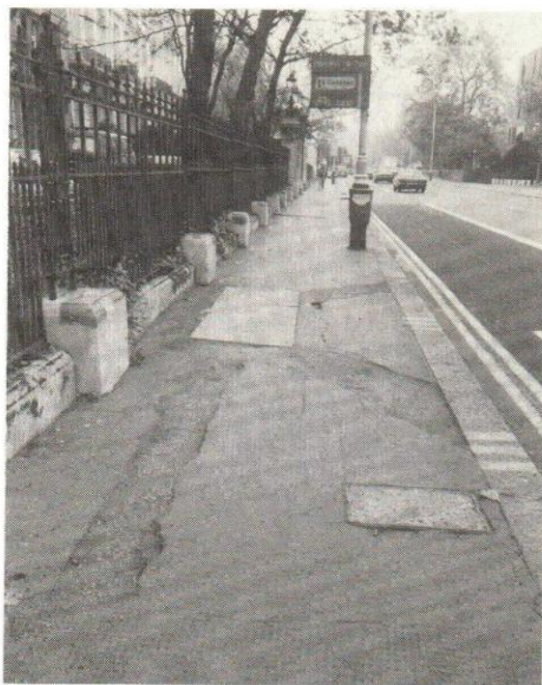
Dangerous paving outside Rutland Court.
