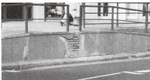
Flaking plaster on the wall of the elevated pavement in Brompton Road.
