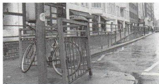
Unsatisfactory split level pavement in Brompton Road, railings need upgrading and co-ordinating, the retaining wall is flaking.
