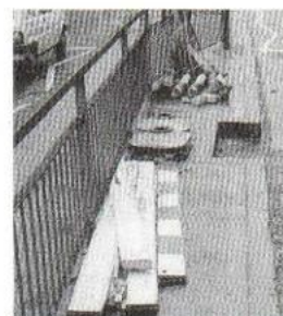
Abandoned roadwork signs on a pedestrian crossing with scattered grit.
