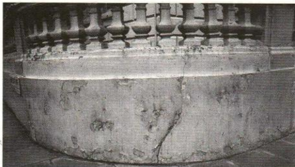
1 Albert Gate, The French Embassy, in great need of repairs and redecoration, adds to the dilapidated appearance of parts of Knightsbridge.
