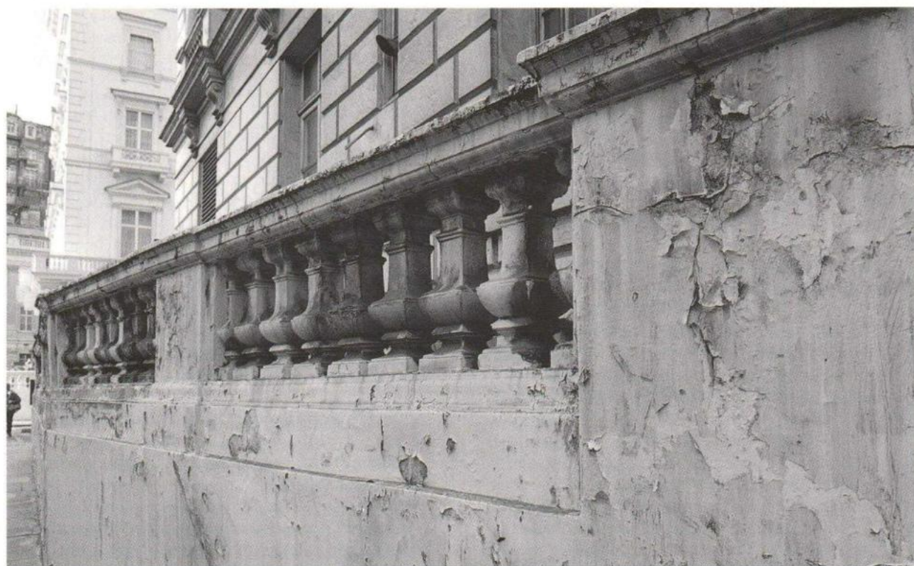
The French Embassy, still cracked and peeling – plus ça change.
