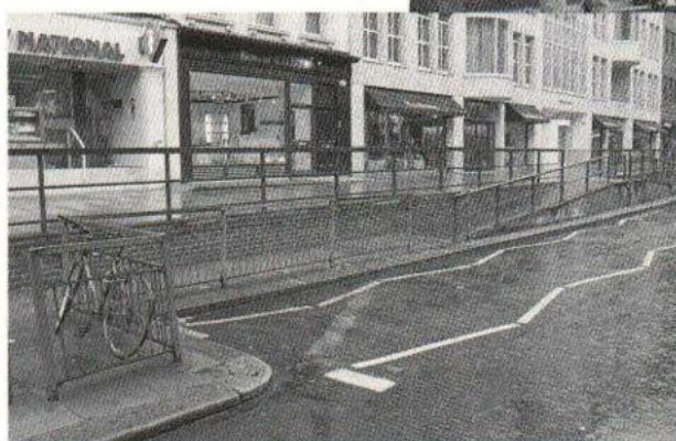
Above: Dilapidated railings in Brompton Road.
