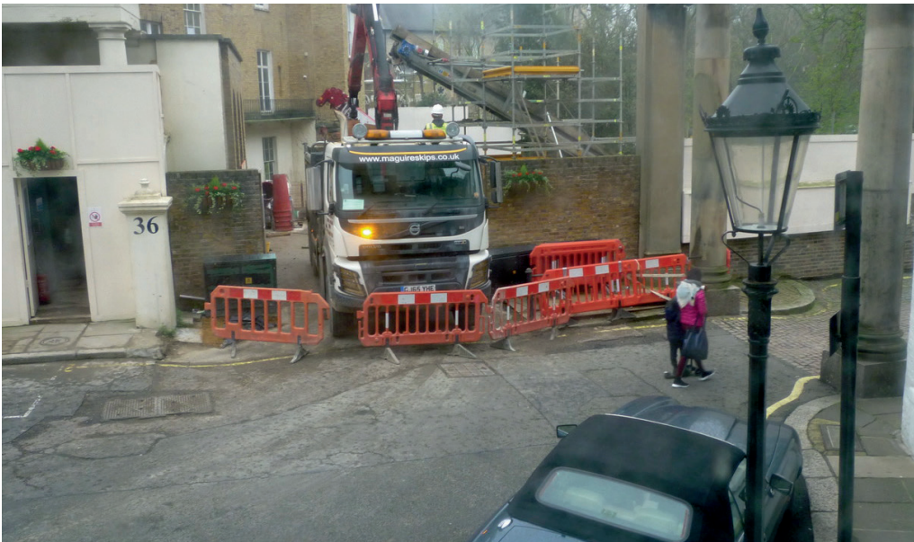
31 Brompton Square. Concerns remain for the stability of the Mews arch and public safety
